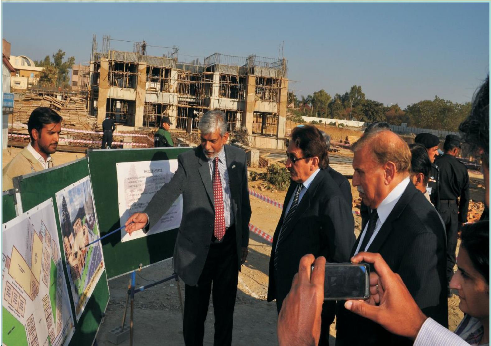
Visit of Hon'ble Chief Justice of Pakistan at Construction site of Federal Judicial Academy, Islamabad
